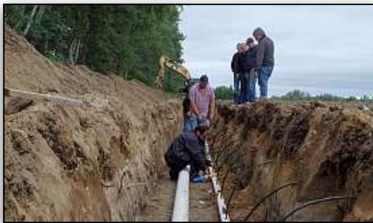
Installing drip lines, one foot deep. (PHOTOS COURTESY OF OSGOODE FARMS LTD.)
