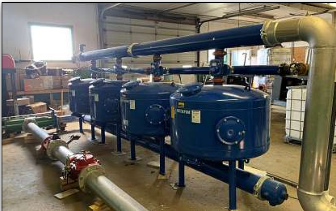
Osgoode Farms has four sand filters.
